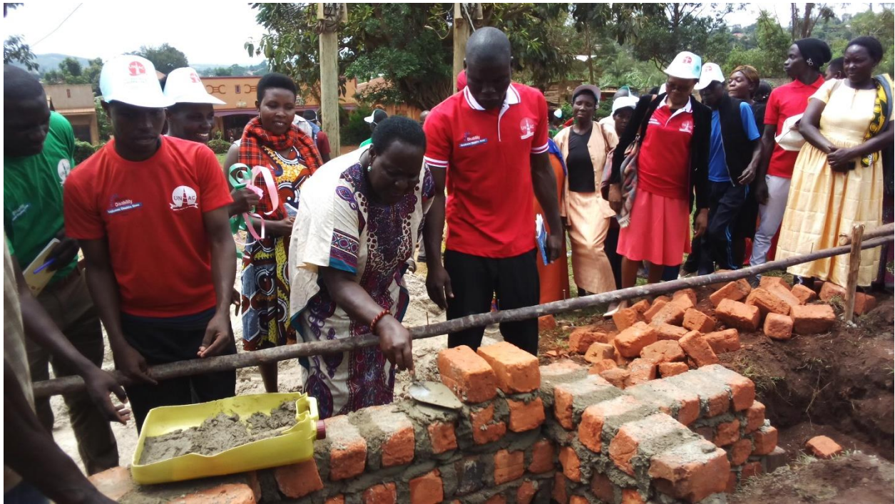
UNAC advisory technical Board and Chairman Board putting a brick on the construction site of UNAC inclusive Day care centre as Executive director, CDO and Parents sees.
